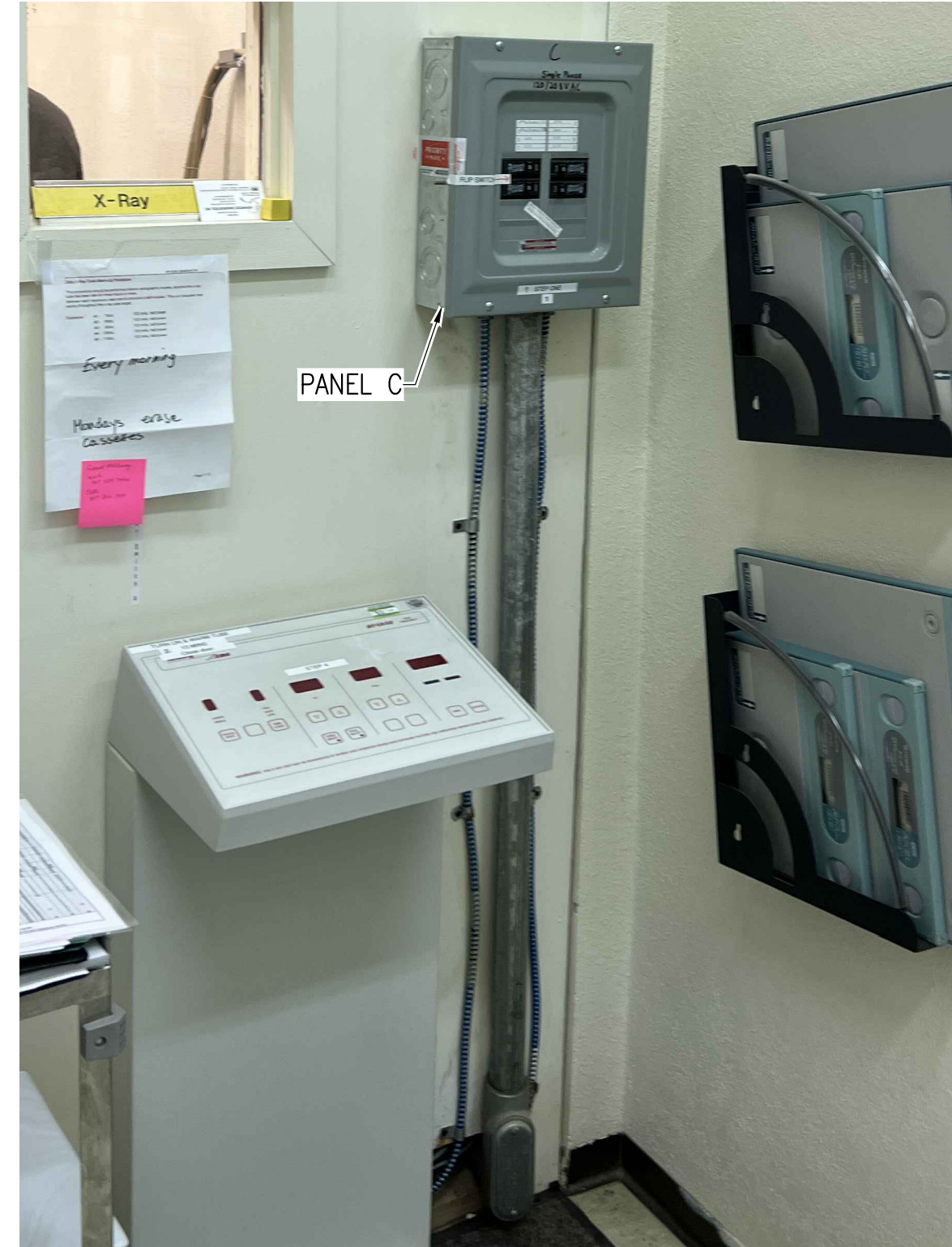
4 PHOTO - EXISTING PANEL C E3.01 SCALE: NONE
