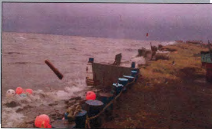
Nelson Lagoon resident Elvis Johnson took photos of the destruction to the wooden seawall during the storm in late October. Photo courtesy: Elvis Johnson.
