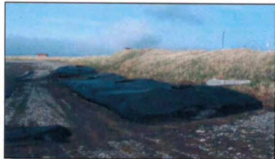
Other erosion control measures included installing a geotube containment structure several years ago.
