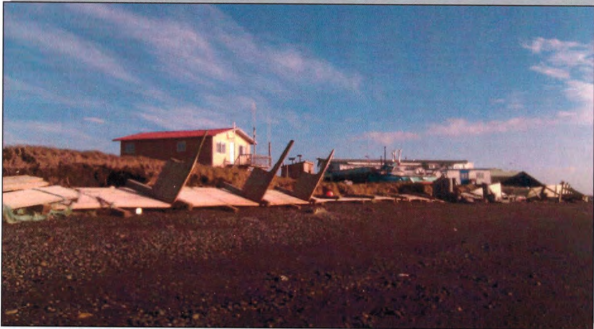
During the storm, the wooden seawall collapsed. “It’s lying flat on the ground. Some of it folded backwards. Some of it folded forward,” McNeley said. Photo by Elvis Johnson.
