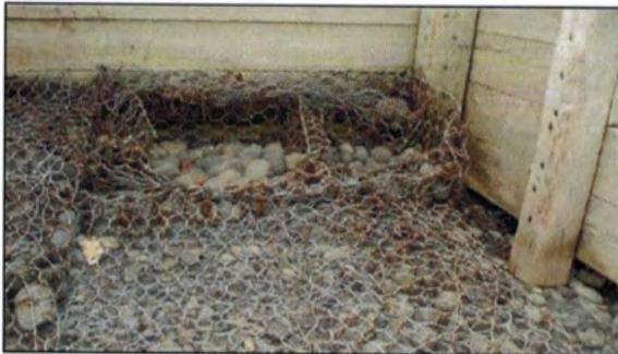
In the past, the community installed gabions behind the seawall to absorb some of the wave energy.
