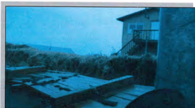
Nelson Lagoon's wooden breakwater was knocked over during the recent storm. Photo by Mark McNeley.
